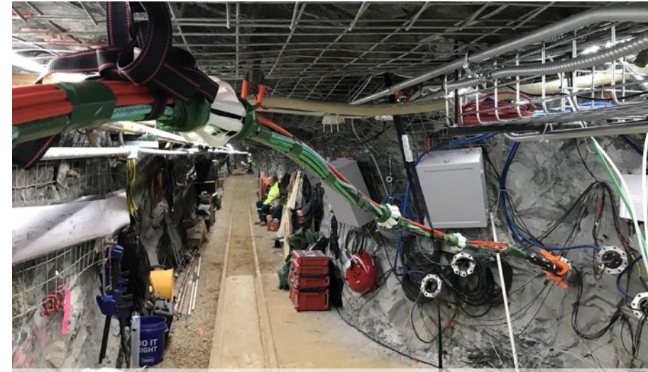
SIMFIP tool installed for EGS/SIGMA-V
