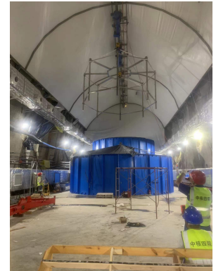
FIGURE 8: Lifting of the upper half of the OSIRIS SS frame into the tank.
