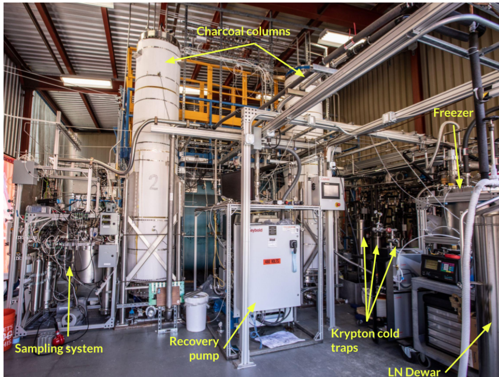
FIGURE 2: Physical layout of the krypton removal system at SLAC.
