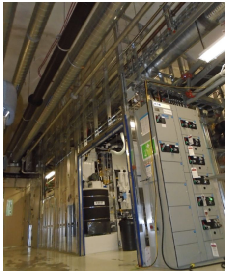
underground TeA purification plant
