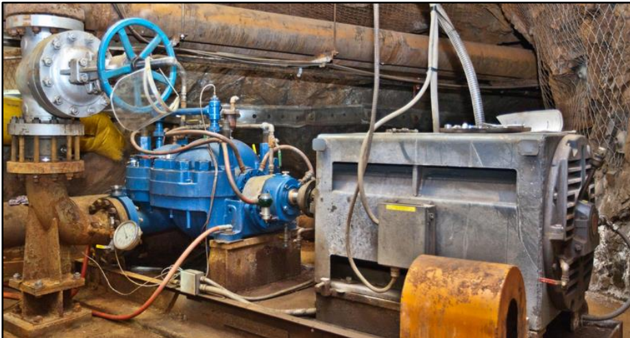
Underground pump station
