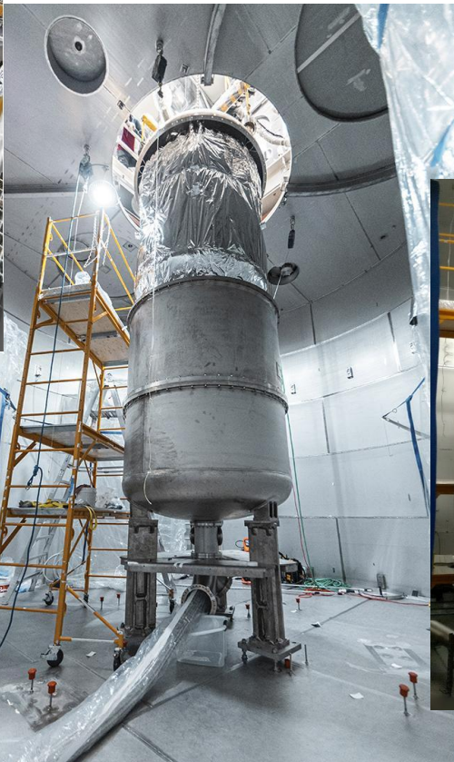
ICV, wrapped in insulation, entering the OCV
